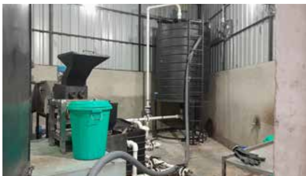
Figure 9: Biogas unit (Distributed Architecture Model) in ward 32, set up by RWA
